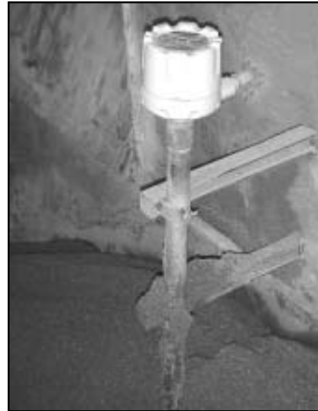
An installed SafePoint ® unit in an aggregate application.
